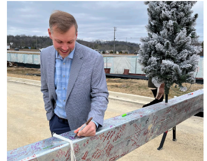
Beau Barth, VP of Operations at McCarthy signs beam. The tree symbolizes reverence for life.
