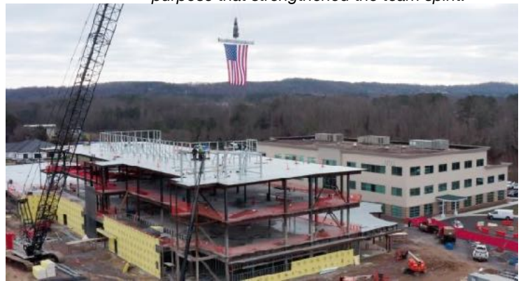
“Looking up at the steel beams, the backbone of this structure, it’s hard not to feel the promise and excitement of the healing miracles that will take place in this sacred edifice.” - CEO Janelle Reilly
